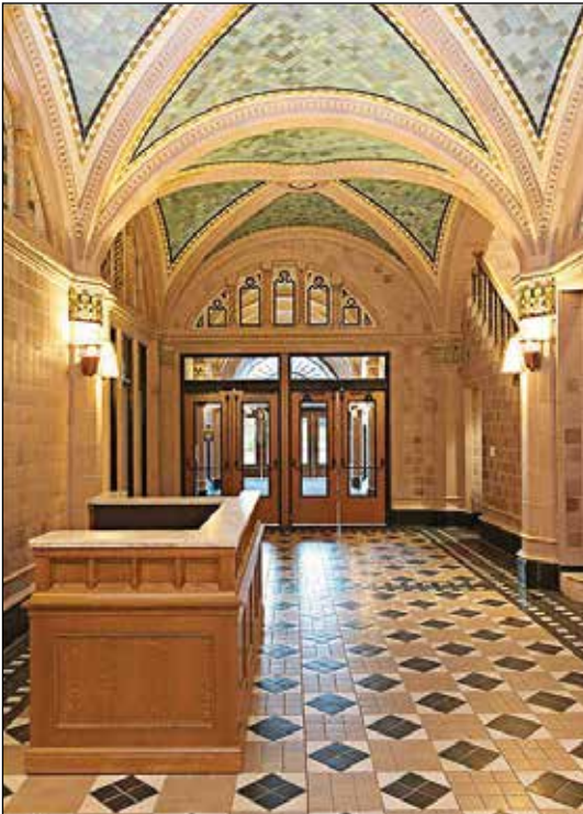
The Monroe Building Restoration included installation of replicated original ceramic tile that was installed 100 years ago.
